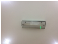
Emergency lighting bulkhead
